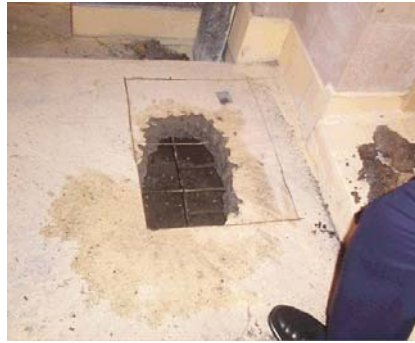
Fig 4. Hole in concrete floor, to destroy termites found with thermal imaging.
