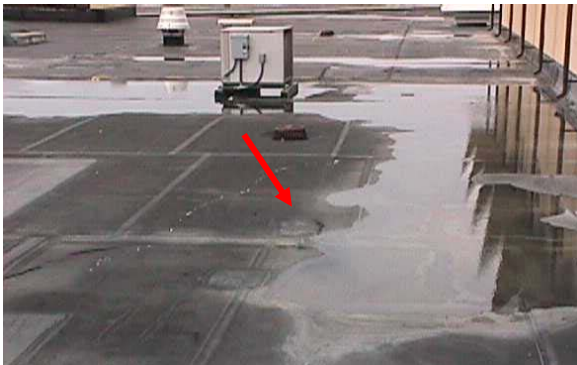
SECTION OF EPDM ROOF WITH STANDING WATER
