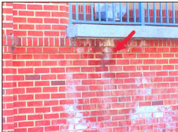
Figure 1. The efflorescence on the exterior walls illustrates the amount of damage that can occur when a problem is left unchecked
